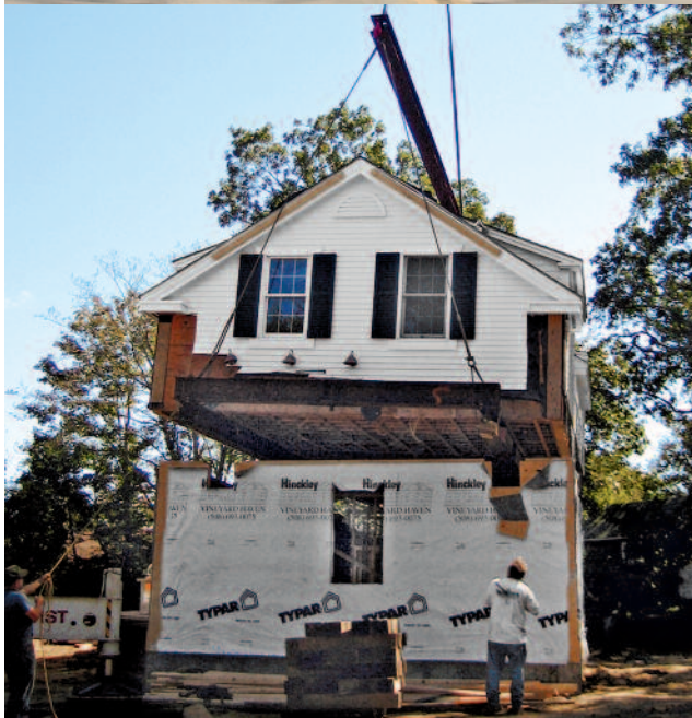
The upper floor of Michael Kidder's Greek Revival house was raised atop cribs, moved on a flatbed, and lowered onto a new first floor.
